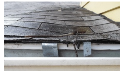
Sagging Shingles or Gutters Pulling Away
